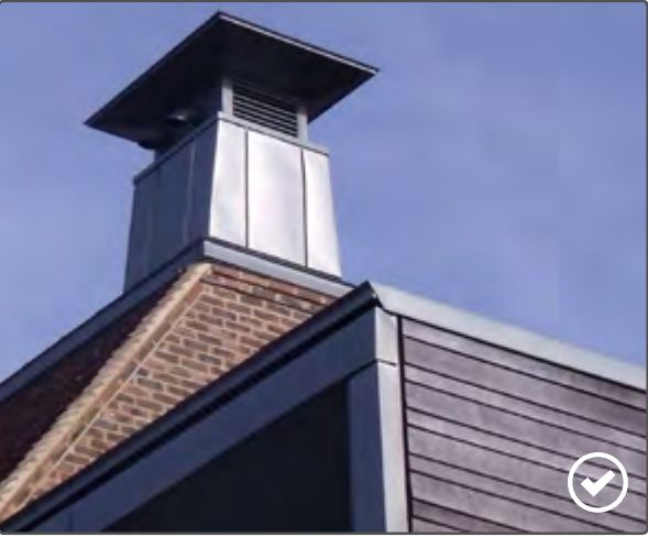
A good example of standing seam used on this ventilation chimney, Cambridge
