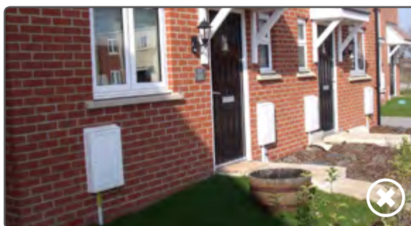
Poorly located meter boxes - St Ives
