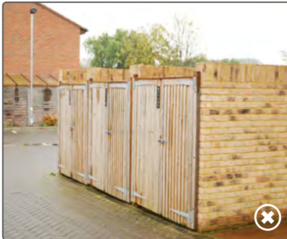
A poorly designed bin enclosure
