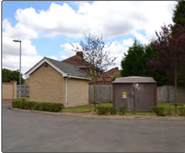
How not to locate or design a substation
