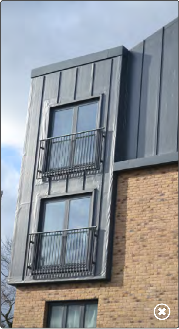
Here we can see this applied material bubbling up
