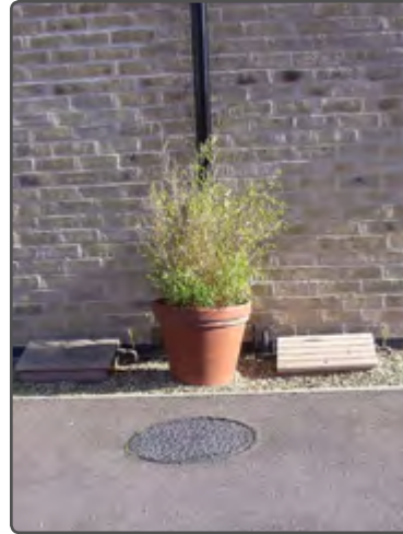
Semi concealed gas meter
