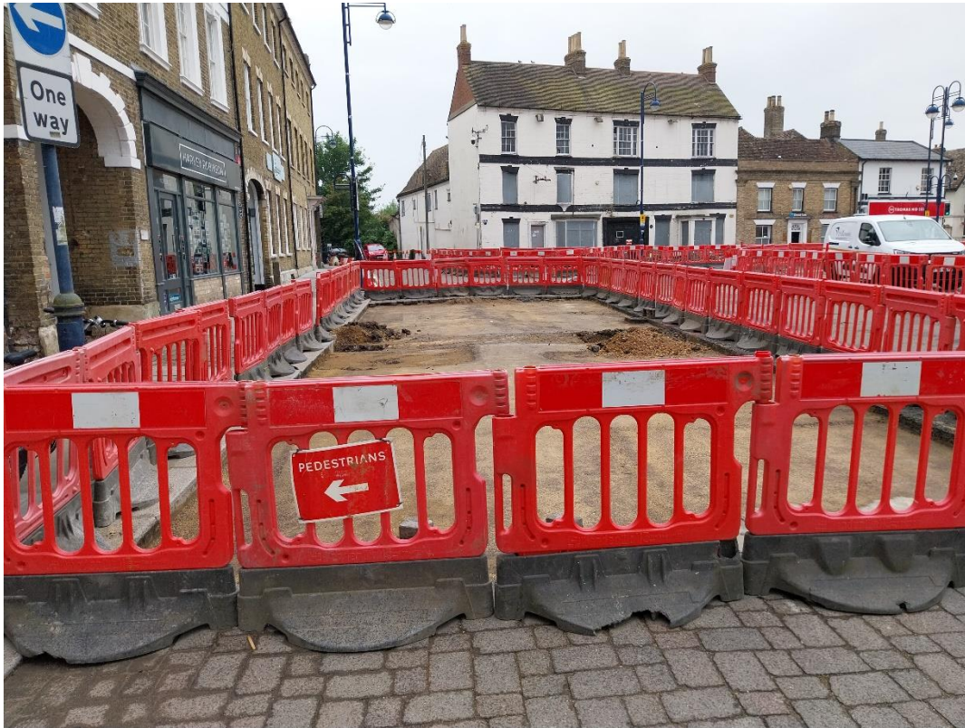
03/07/24 – Relaying of Market Place continues. Next section has been stripped ready for kerb line excavation, installation and relaying of the carriageway blocks.
