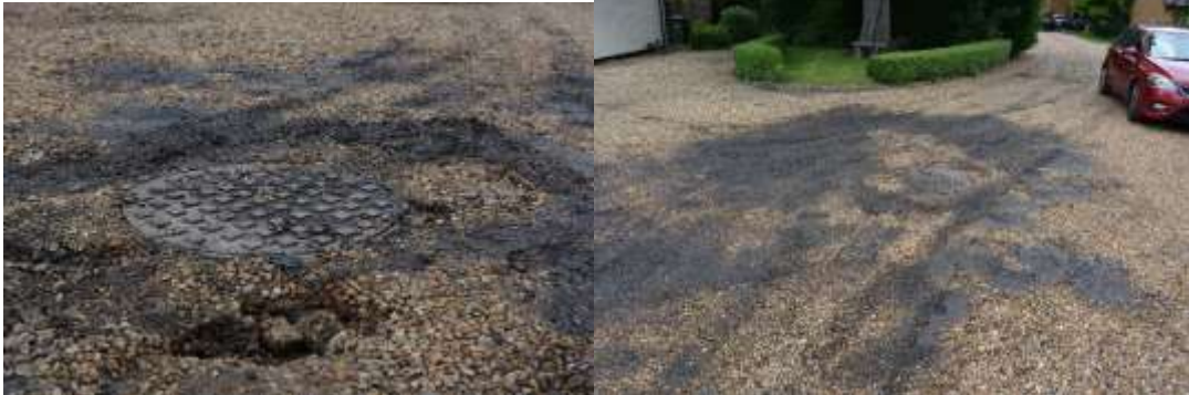
Figure 61: Flood damage in Ellington in June 2014
