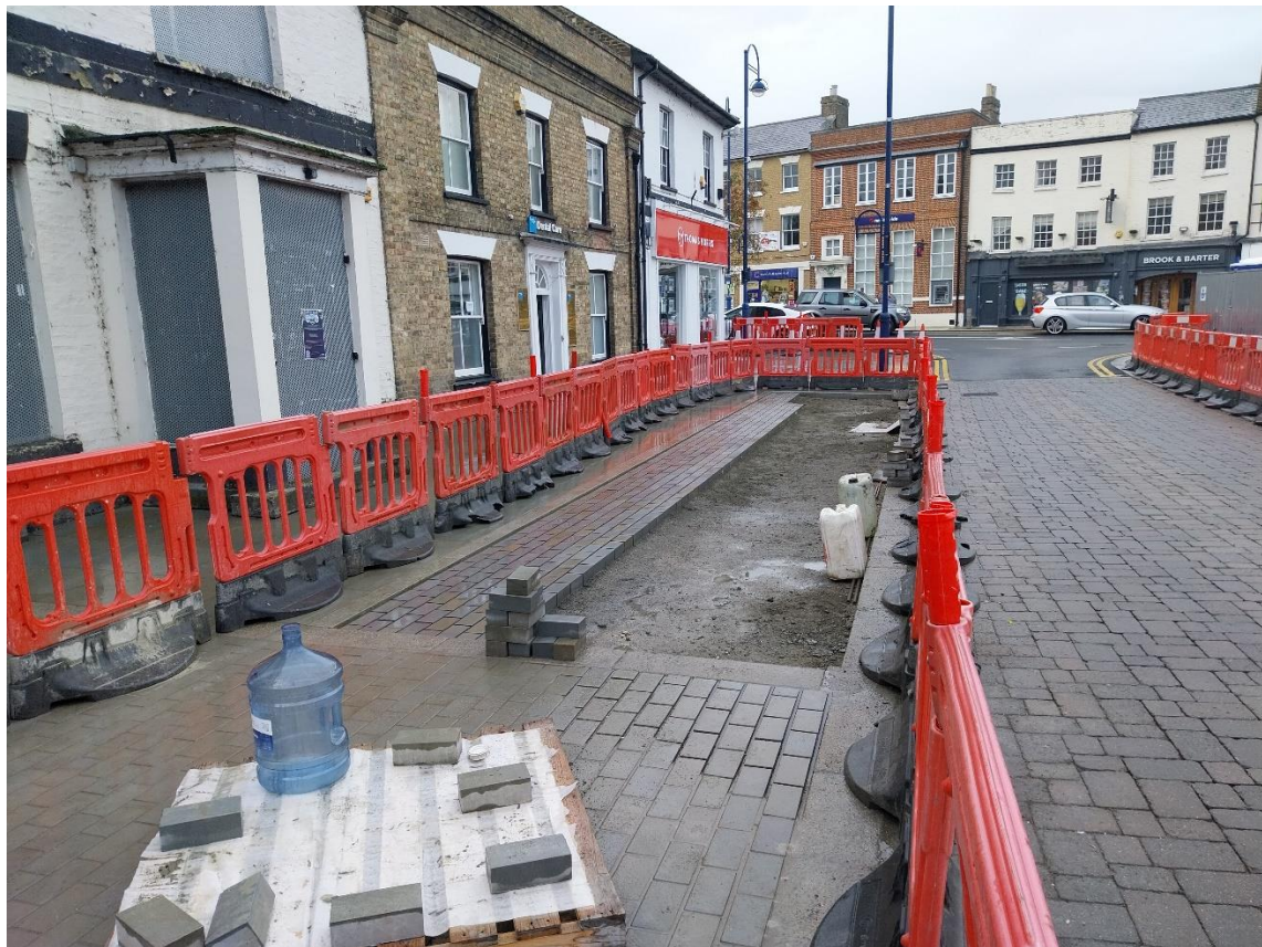
09/10/2024 – Pavement and access renewed outside the Old Falcon, loading bay slab-laying in progress
