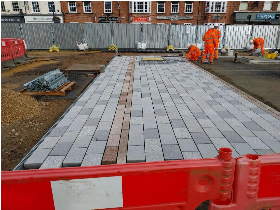
09/10/2024 – Slab laying has begun on the north side of the Market Square
