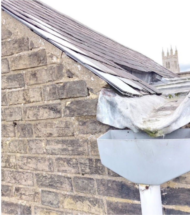
Damage to roof tile Holland and Barratt St Neots
