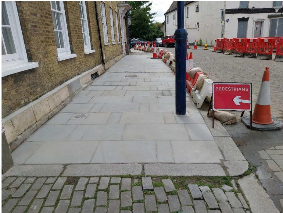
19/06/24 – New Yorkstone paving laid in footways on south side of Market Place. Once the footways are completed, repaving of vehicle accesses along this section will commence.
