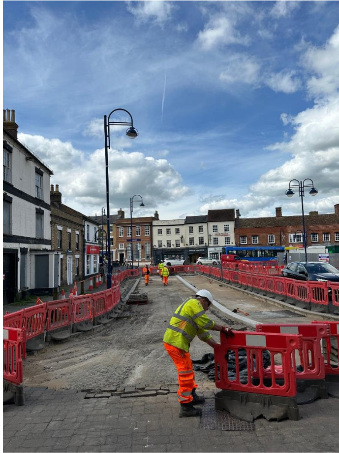
19/06/24 – First section of Market Place stripped, new kerb line installed and subsurface prepared for relaying of blockwork (to commence 20/06/24)
