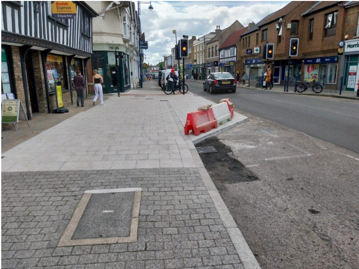
19/06/24 – Footway widened at Church Walk crossing to improve visibility and safety for crossing users
