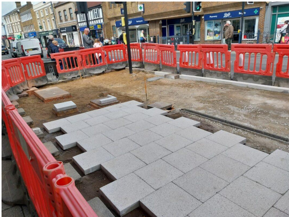
15/05/2024 – Widened footway at Church Walk crossing nears completion. New drainage has been installed and slab laying is in progress. Widening this footway improves visibility at the crossing, increasing safety for users.
