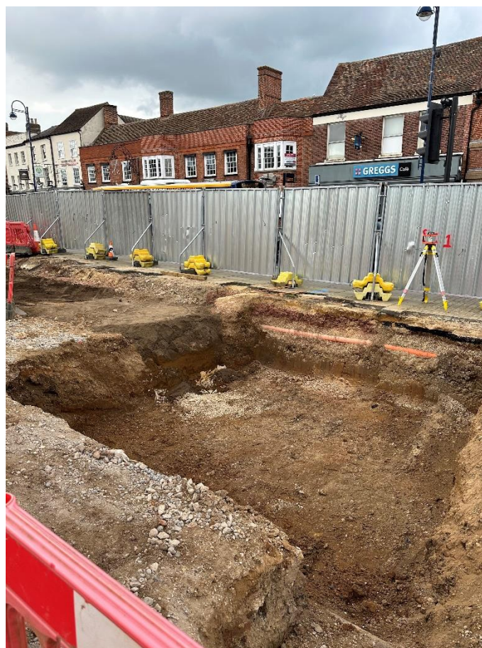
15/05/2024 – Excavations for tree pits, rain gardens and service ducts continue on the north side of the Market Square.
