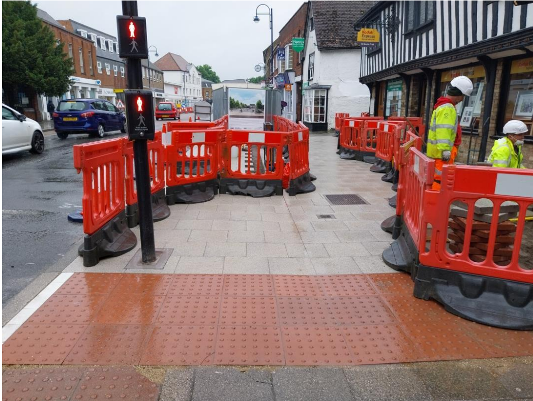
22/05/2024 – Widened footway at Church Walk crossing nears completion. New drainage has been installed and slab laying is in progress. Widening this footway improves visibility at the crossing, increasing safety for users.
