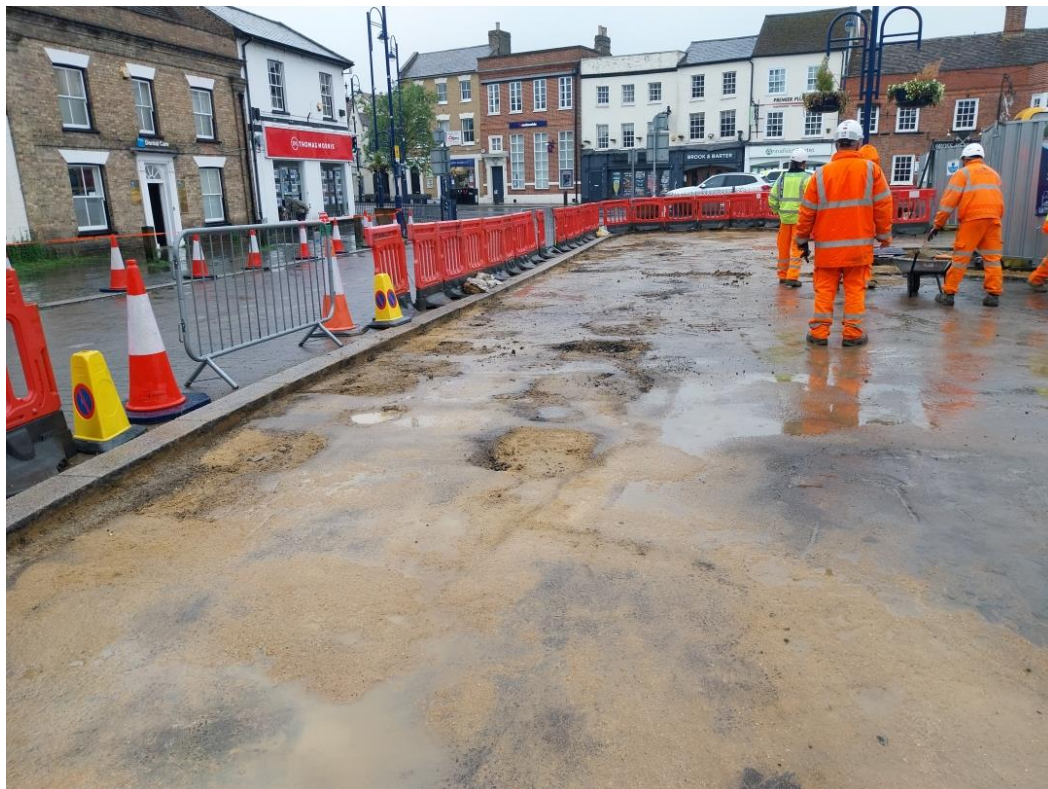
22/05/2024 – Paving removed in footway on west side of the Market Square. The kerbline will be removed and moved to expand the square outwards.
